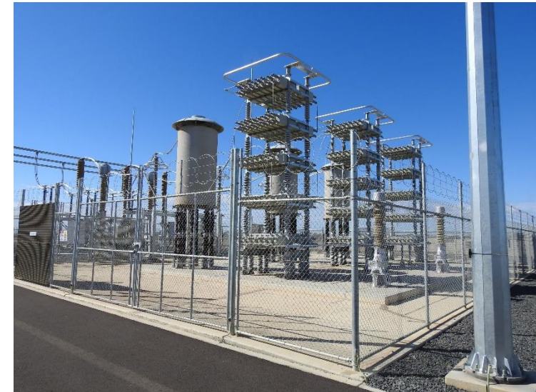
100 Mvar 275 kV capacitor
